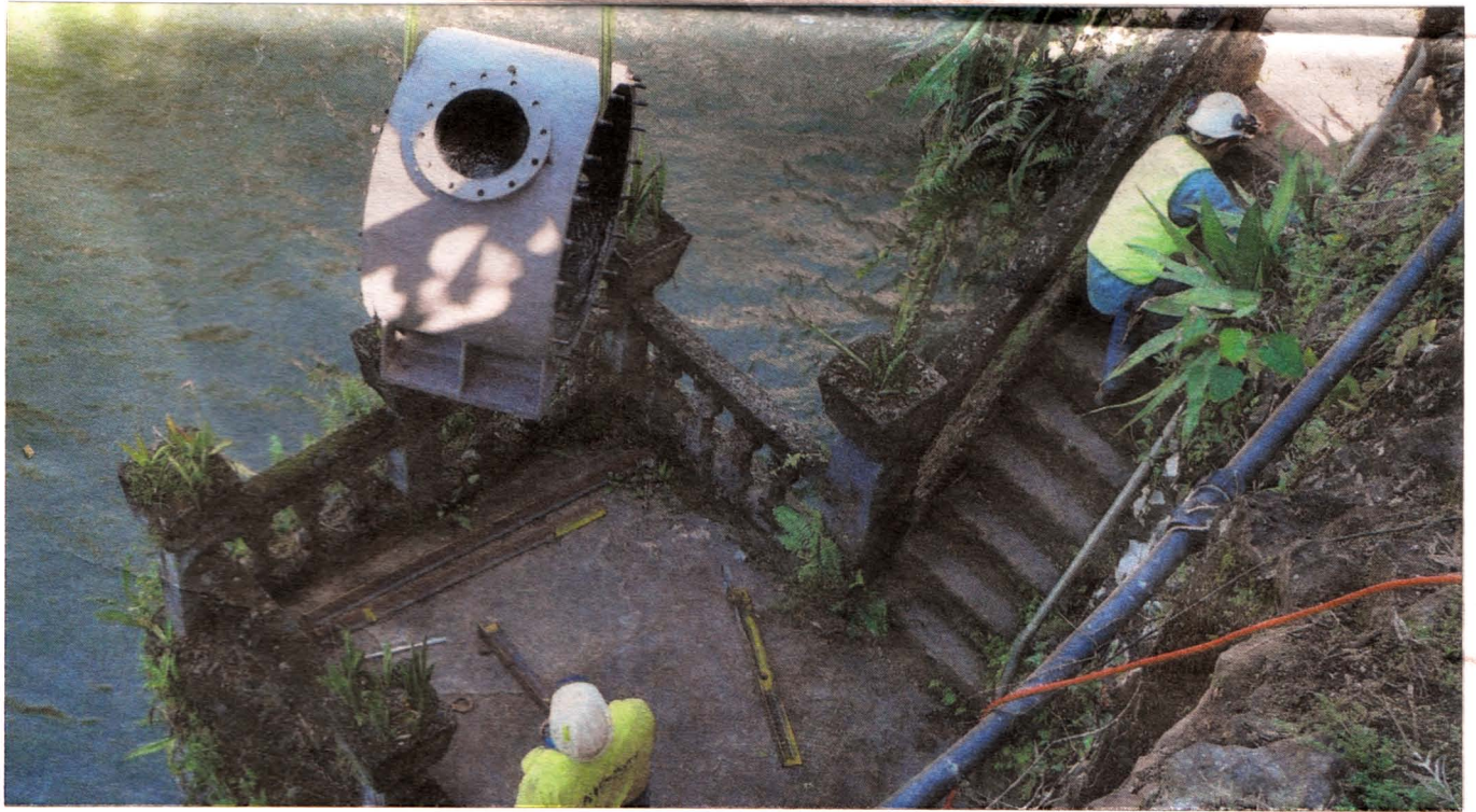
Back in place: Workers lower the 1933 turbine, which was repaired in Germany, into place at Paronella Park yesterday.
